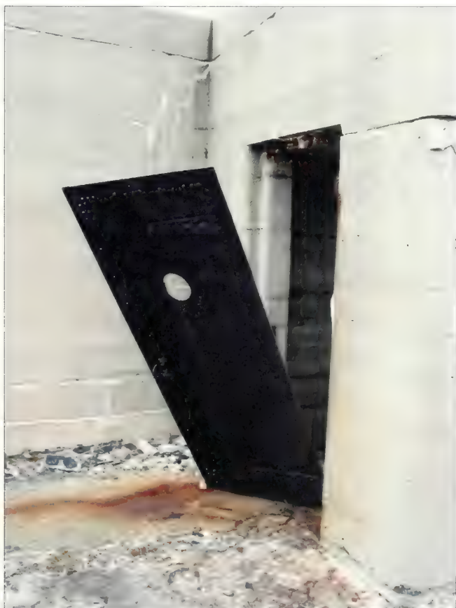
Figure 5.47. View of failing metal door, Nine Gun Battery. Doors and windows should be properly mounted and locked to prevent unauthorized access to interior spaces. While the door in view may be repaired, when a door is damaged or severely deteriorated, a new door should be fabricated to match the existing in materials and finish (Olmsted Center, January 2009).
